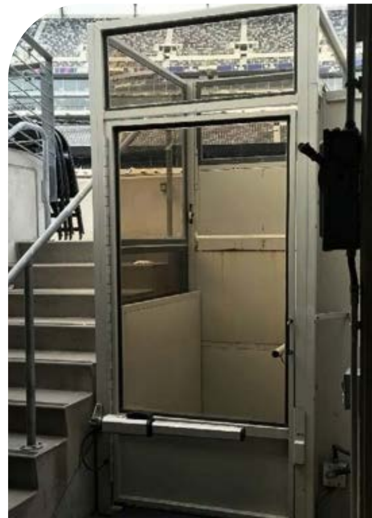
Image 11 | An enclosed platform lift at MetLife Stadium in New Jersey
