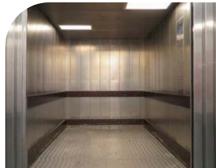
Image 9 | Accessible lift at the National Stadium of Wales
